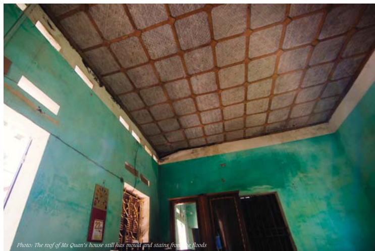
Photo: The roof of Ms Quan's house still has mould and stains from the floods
