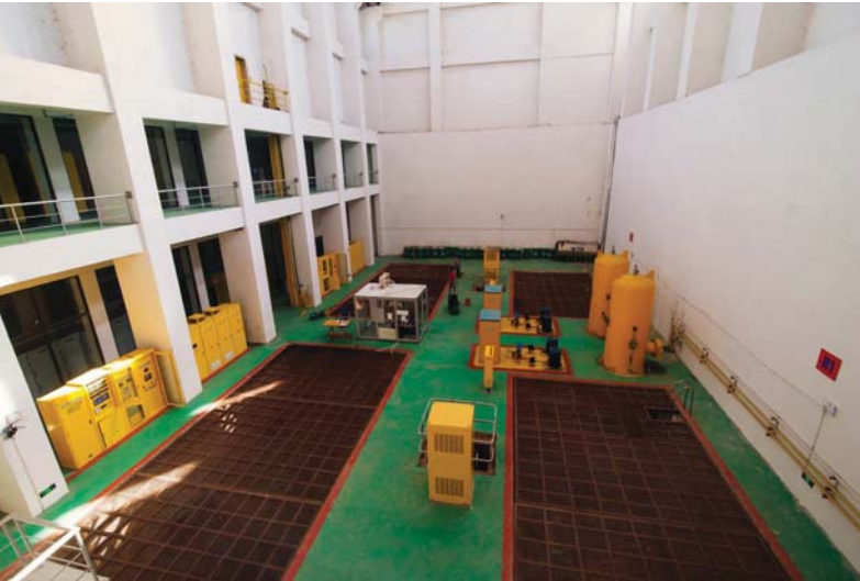
Photo: Inside the Cam Thuy Hydropower Plant 1
