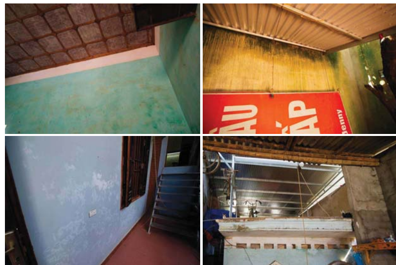
Photo: The walls with flood water stains
